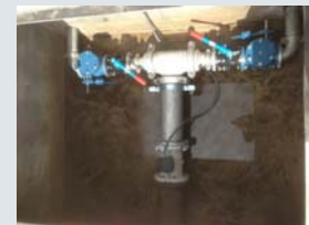
New Stainless Pipe and Valve
