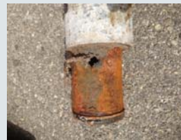
Old Corroded Pipe
