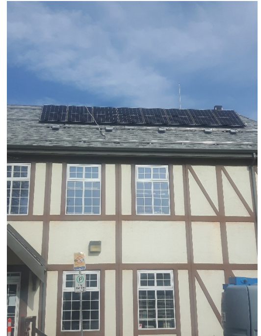
Solar photovoltaics (PV) being installed on Municipal Hall. Source: District of Summerland
