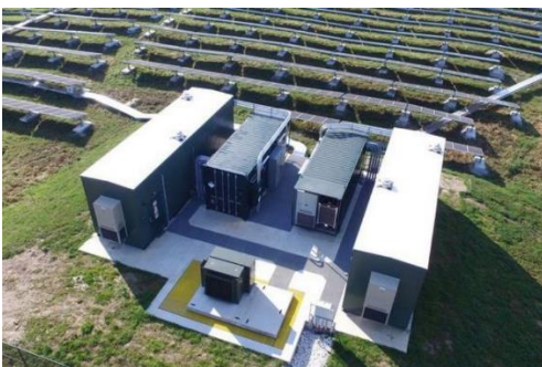
Example solar farm with battery storage. Source: District of Summerland
