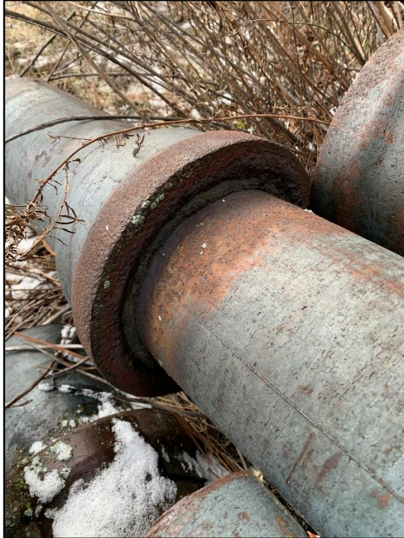
Photograph 5: View of the Suspect Asbestos Containing Pipe Gaskets (December 3, 2019).
