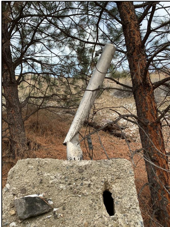
Photograph 6: View of suspected lead pipe located along the north boundary of APEC #4 (December 3, 2019).
